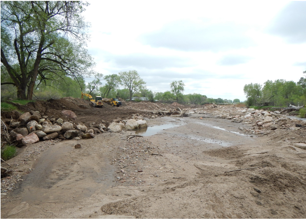
Lefthand Creek flood restoration project, before and after photos, taken May & July of 2014.
