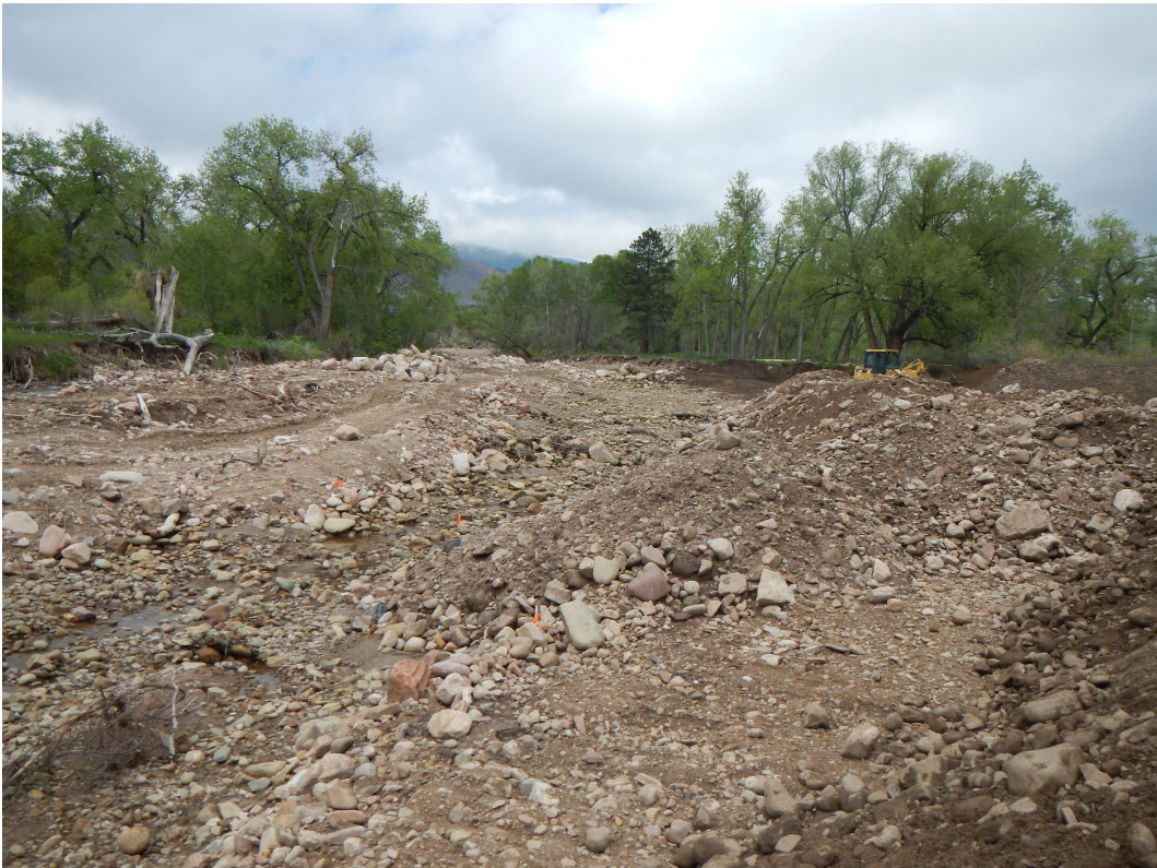
Lefthand Creek flood restoration project, before and after photos, taken May & July of 2014.
